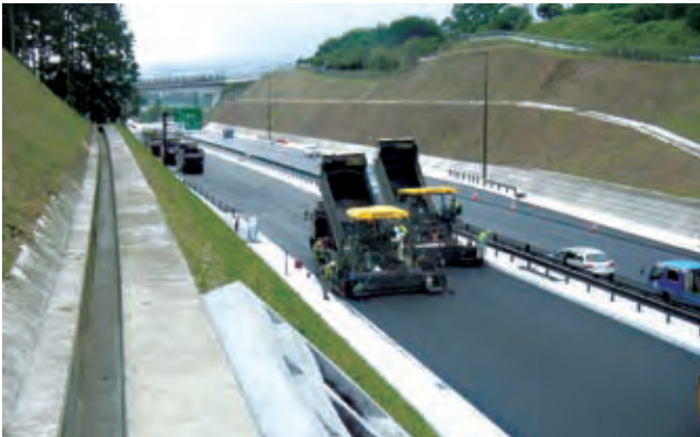
Road paving work on the Izu Jukan Tokura Road (Constructed by Kajima Road Co., Ltd.)
