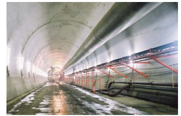
A belt conveyor installed within the Hakkoda Tunnel worksite
